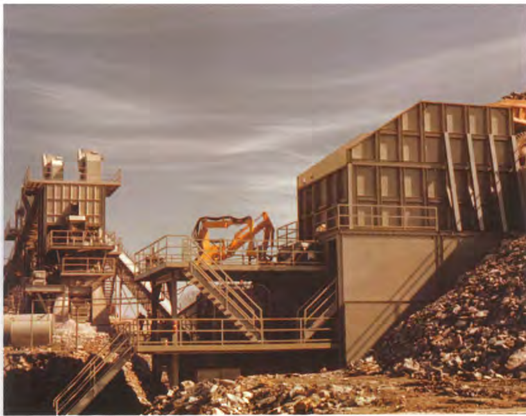
Opened in 1972, this quarry in Hopkinsville, Kentucky, continues the Rogers tradition of maintaining an orderly workplace.
